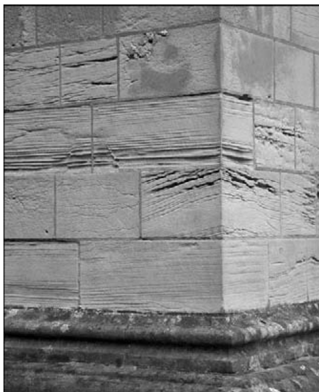
Thirteenth Century exterior work in Mansfield Woodhouse stone, with barite mineralisation visible top centre.
