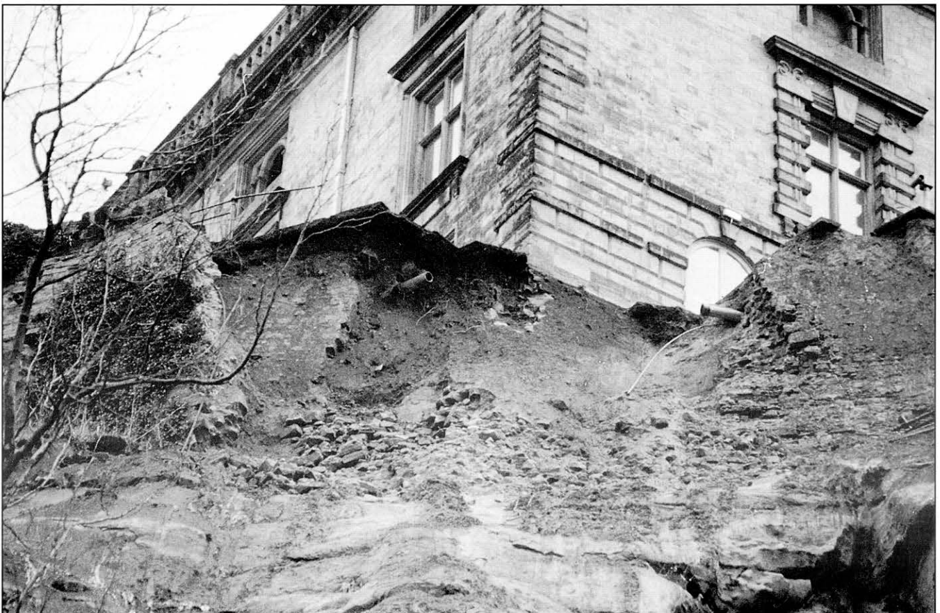
Closer view of the slide scar, with the masonry of the Norman wall visible beneath the overhanging terrace paving; undisturbed sandstone is exposed at the foot of the picture.
