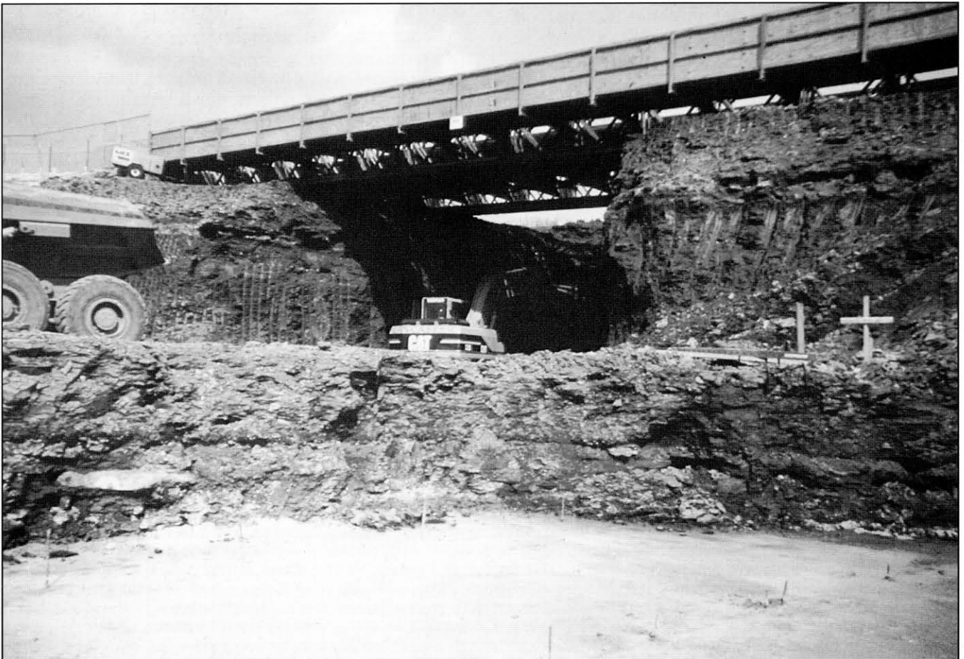
Fig. 2. Temporary overbridge of A607 road, supported on the Marlstone Rock Formation (upper strata) overlying Brant Mudstone Formation. The concreted foundation for the permanent bridge is in the foreground.
