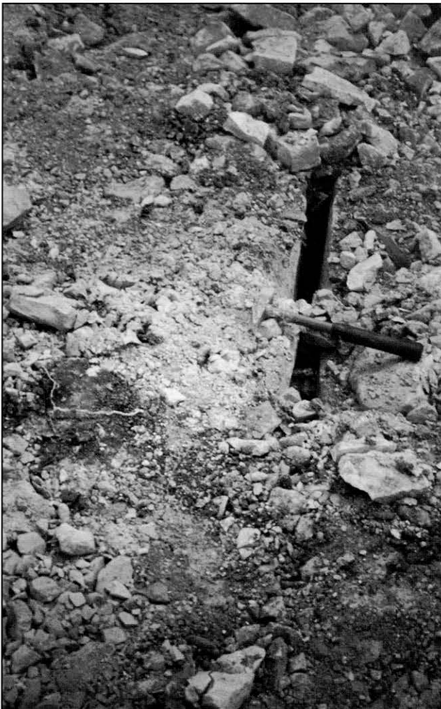
Fig. 7. Joints up to 100mm wide in Lincolnshire Limestone. These trend parallel to the valley side at the top of upper escarpment, and have opened up as a result of cambering of the Limestone.
