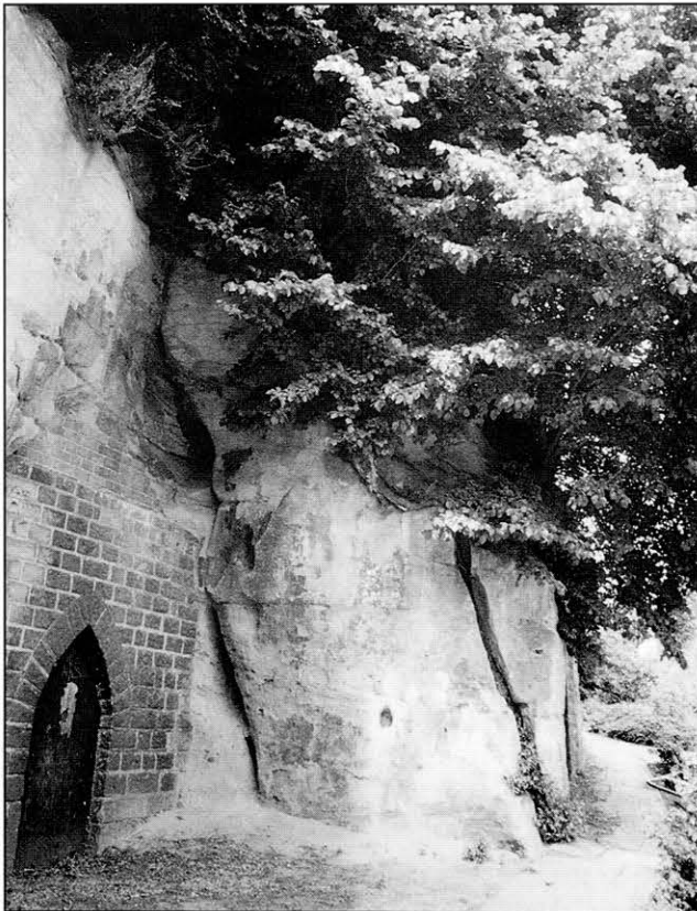
Fig. 4. The widening fissure beneath the unstable sandstone slab beside Castle Road, before the trees were removed and the rock was bolted.
