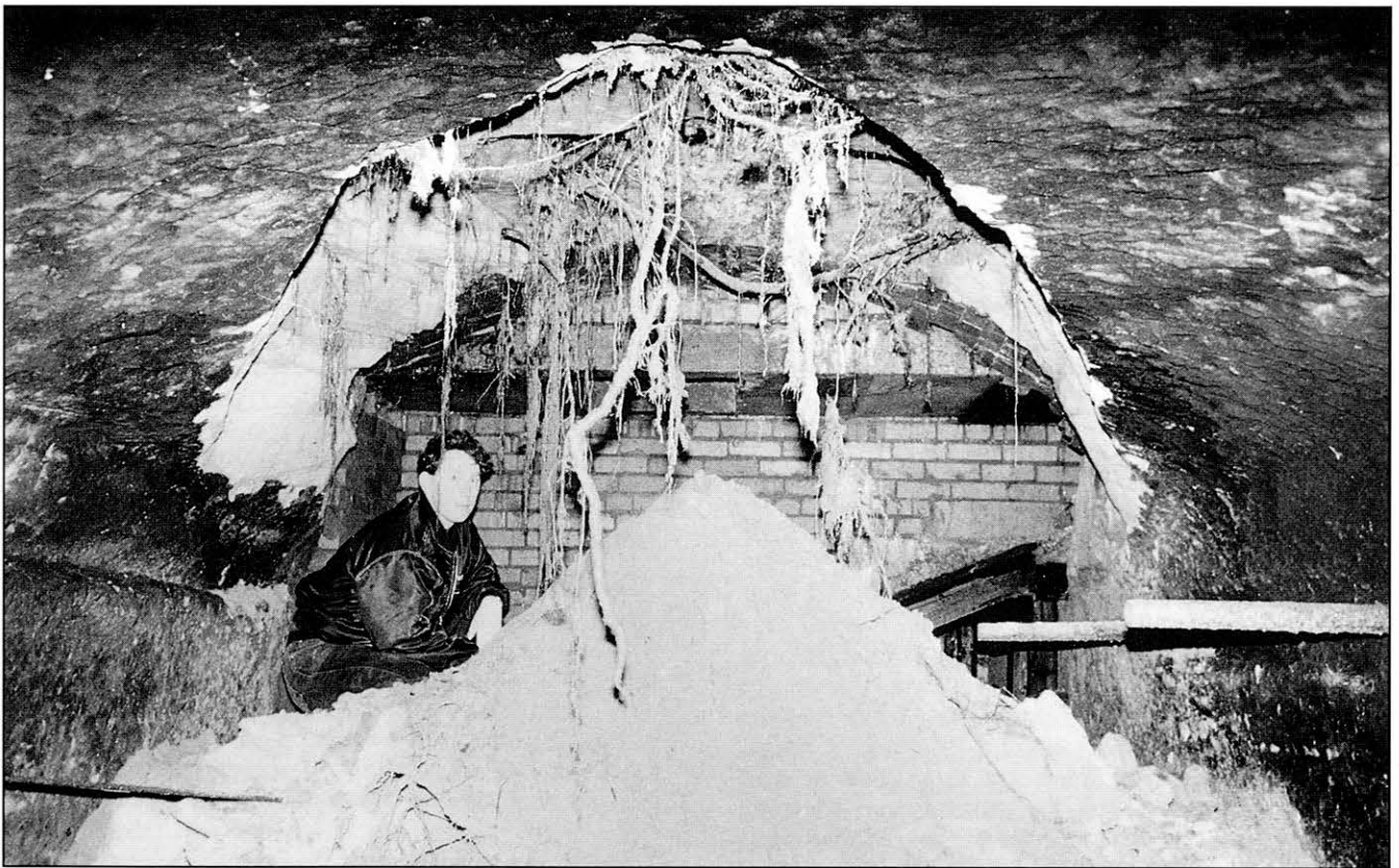
Fig. 3. Tree roots hang from the failure zone where a crown hole developed beside North Sherwood Street. The roof sandstone was little more than 1 metre thick, and tree roots had grown into it from a thin soil cover. The fallen debris on the floor is broken blocks of sandstone capped by a cone of completely weathered sand and soil. The brickwork in the background is not related to the failure (photos by Tony Waltham).
