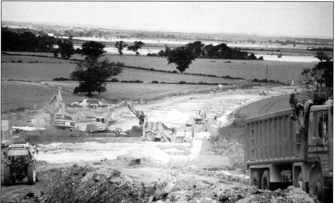
Fig. 6. Installation of the drainage system to de-water head deposits before construction of the embankment.
